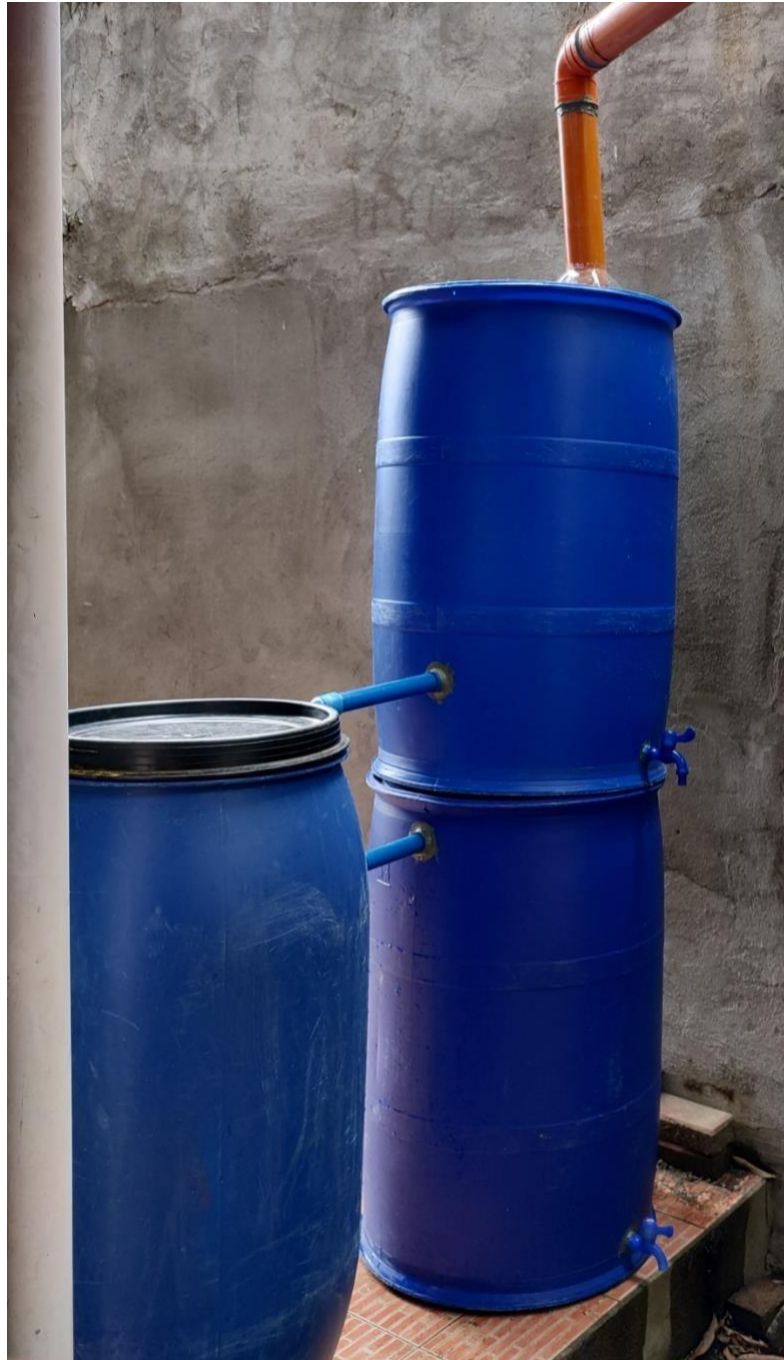
Figure 4 The installed eco-raincatcher
